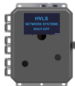
Fire Panel with Wireless Module
